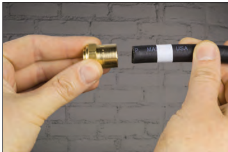
3 Mark the point of full hose insertion depth with a piece of tape.
